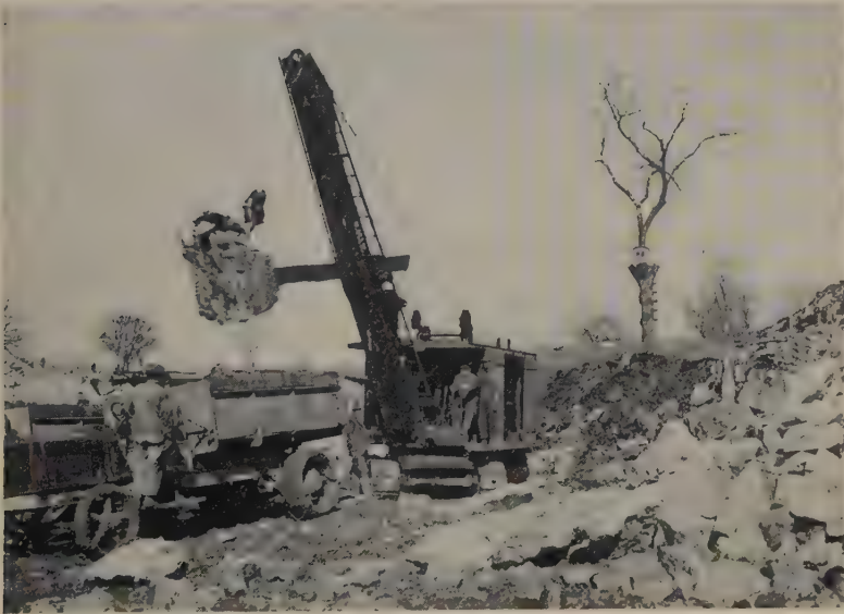
A clear example showing how the inventive genius of Builders serves to replace manual labor. The same work is being accomplished in each case.
